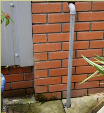
Unprotected metallic pipework exiting the ground.
