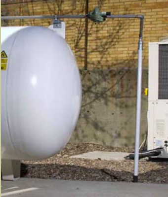
PE protected pipework exiting the ground.
