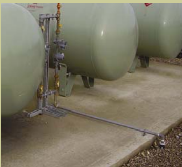
PE protected pipework entering the ground.
