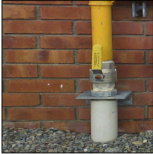
Protected PE exiting the ground
