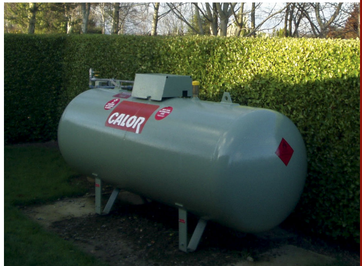
A Calor bulk tank provides all of the gas required.
