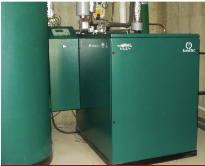
The Calor powered CHP system delivers a constant 5.5kW of electricity and 12.5kW of heat.
