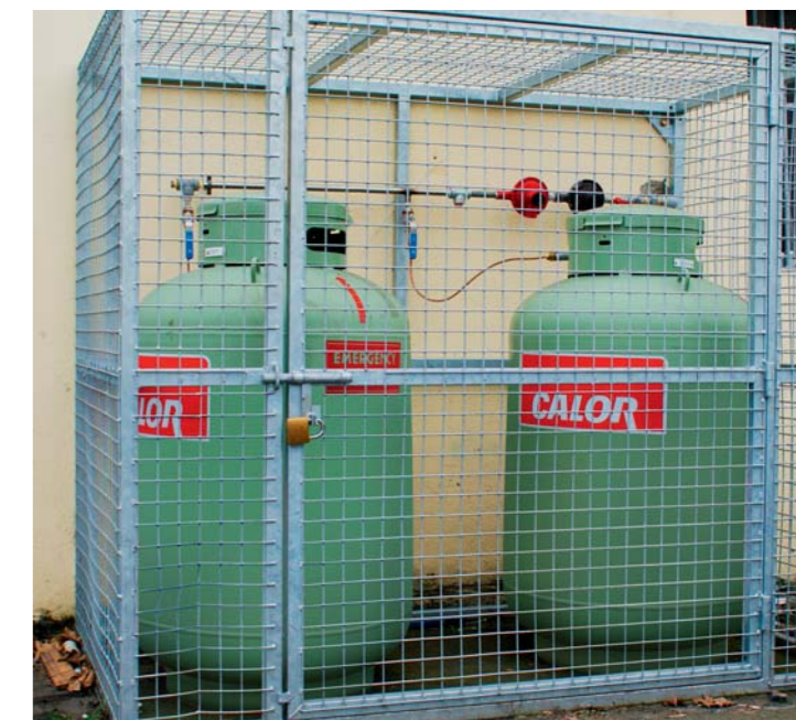
Two 450Ltr mini bulk tanks located in the store car park.
