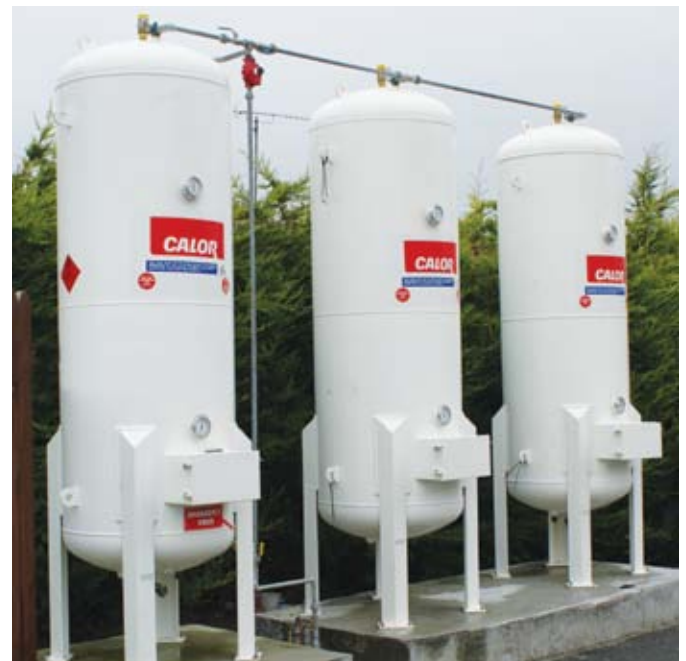
Three Calor 3 Tonne bulk tanks provide a plentiful supply of LPG for all of the Nursing Home's requirements.
