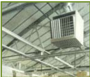
Direct fired heaters heat areas of high ventilation
